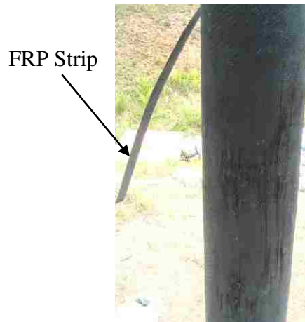
Figure 6.8. Damage to Column 3 after 2 nd 4 lbs Blast
