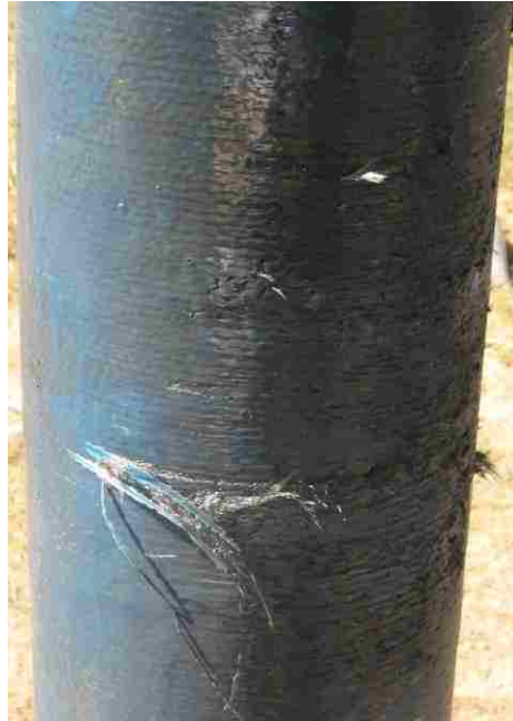
Figure 6.4. Damage Area of Column 2 after 1 st 4 lbs Blast
